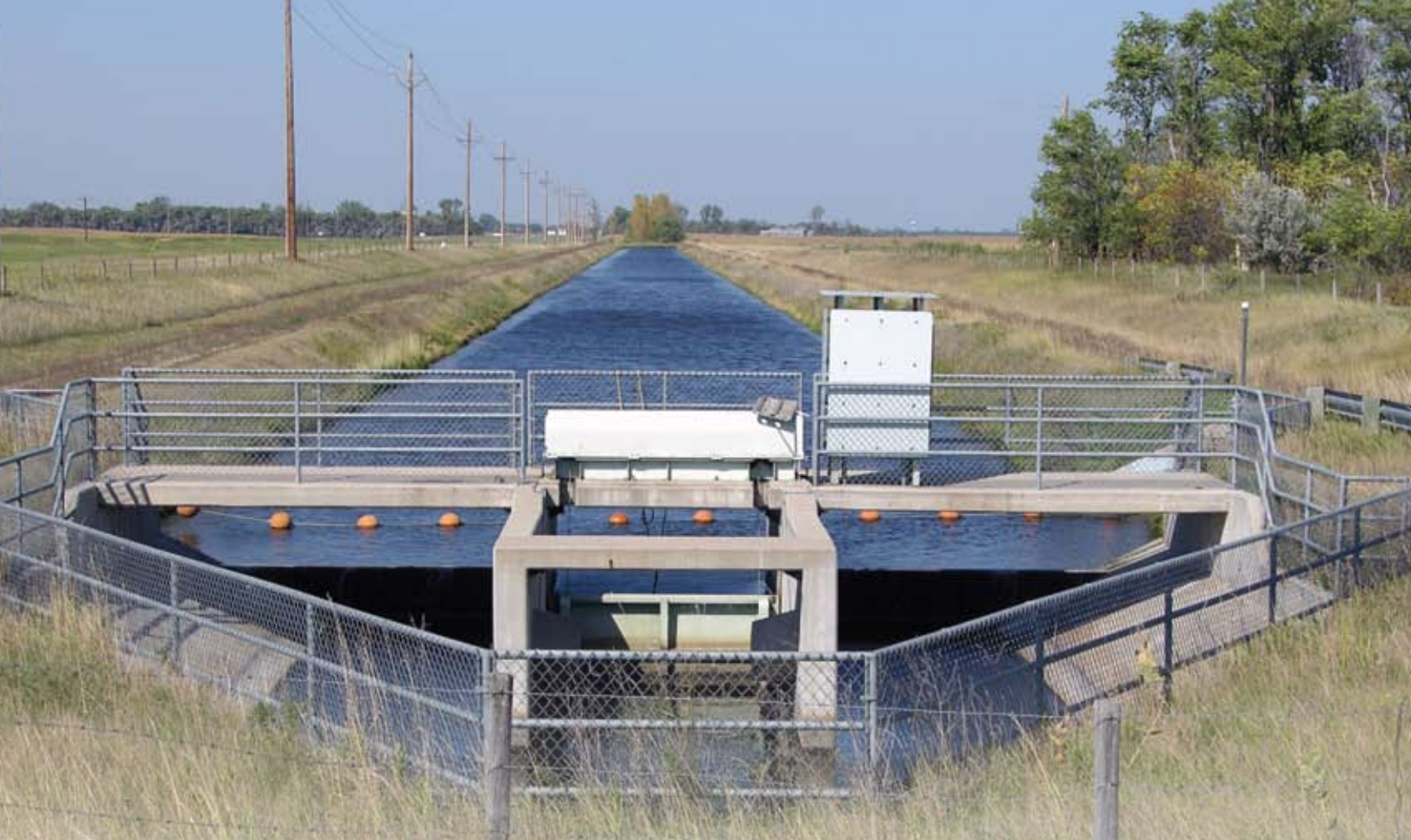
This radial gate maintains flow on the Oakes Test Area Lateral 0-2.0. Water then flows via gravity to pumping plants, which deliver water to irrigators' fields.
