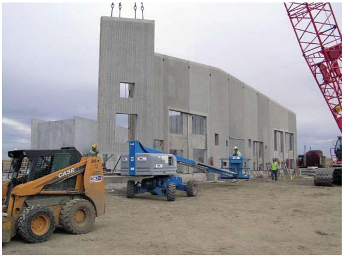
This photo shows equipment placing the pre-cast panels for the Emmons County water treatment plant, which will provide service to 650 homes in Burleigh, McLean, Kidder, and Emmons counties.
