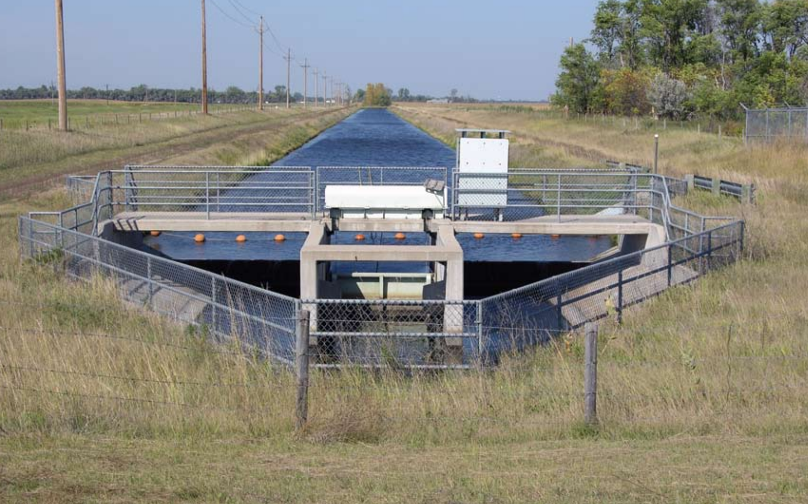
A radial gate structure on the Oakes Canal.
