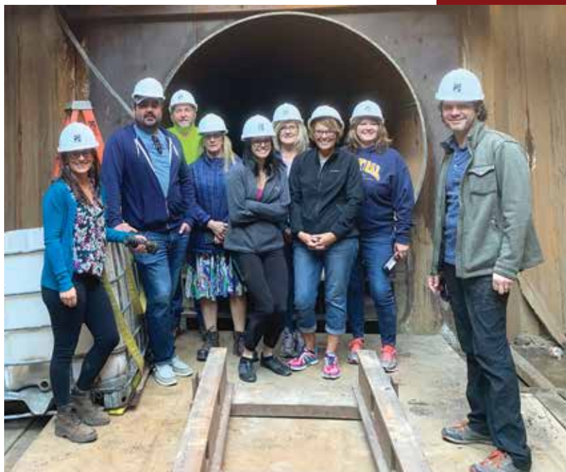
Garrison Diversion staff took the opportunity to walk through the tunnel under U.S. Hwy 52/281 and the RRV/Western Railroad, where the 72" pipe will be placed. The excavation pit is approximately 20 feet deep. Staff is pictured in the jacking pit at the entrance of the pipe.
