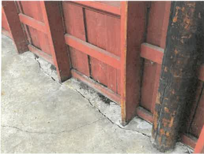
Some Floor Cracks, Nothing Structural
