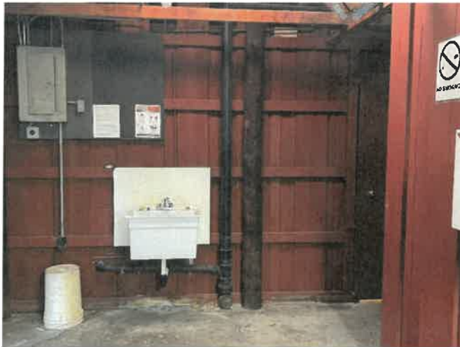
View of Utility Sink and Electrical Panel
