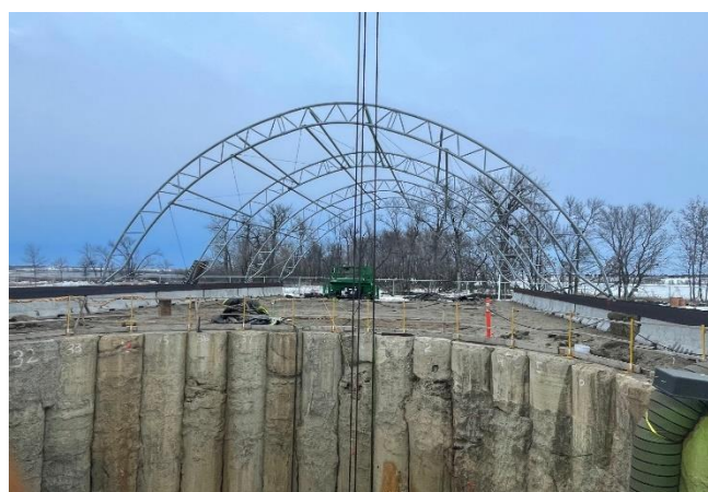
Winter Enclosure Structure
