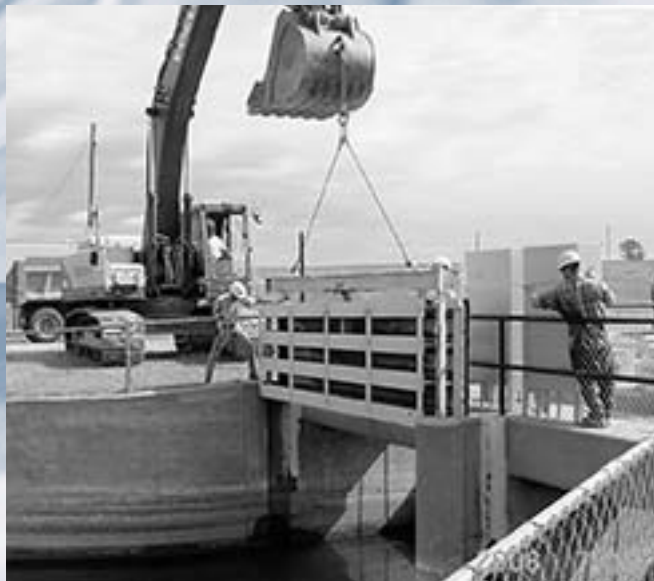
O&M workers placing north stoplogs at New John's Lake for canal pumpdown
