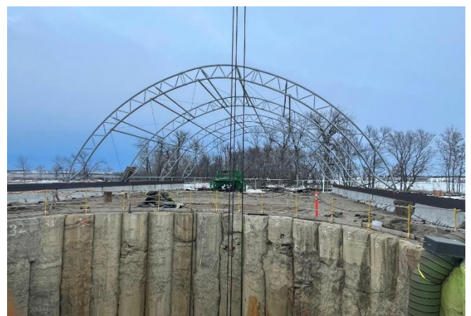
Winter Enclosure Structure
